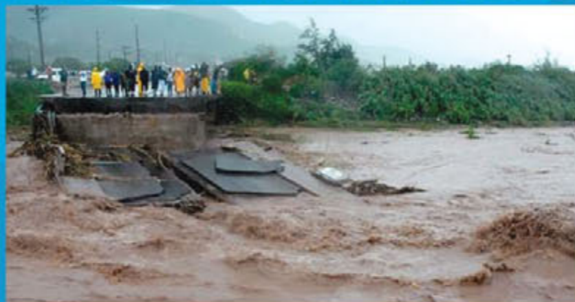
The obliteration of the bridge that connects Kingston to St.Thomas by the raging waters of the Hope River after Hurricane Gustav made landfall in Jamaica in 2008.
